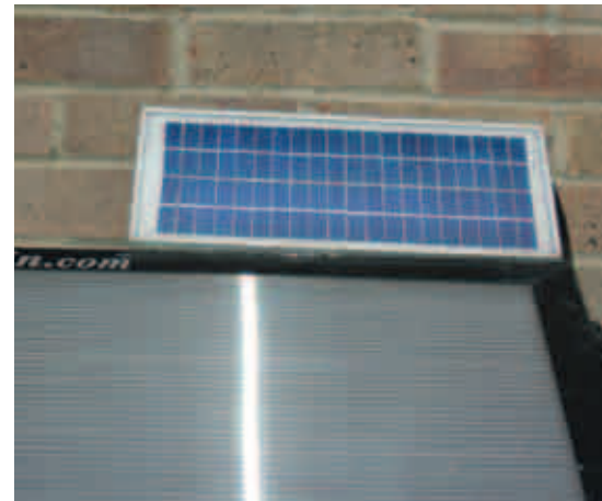
The photovoltaic panel that powers the whole system mounted above the solar panel
