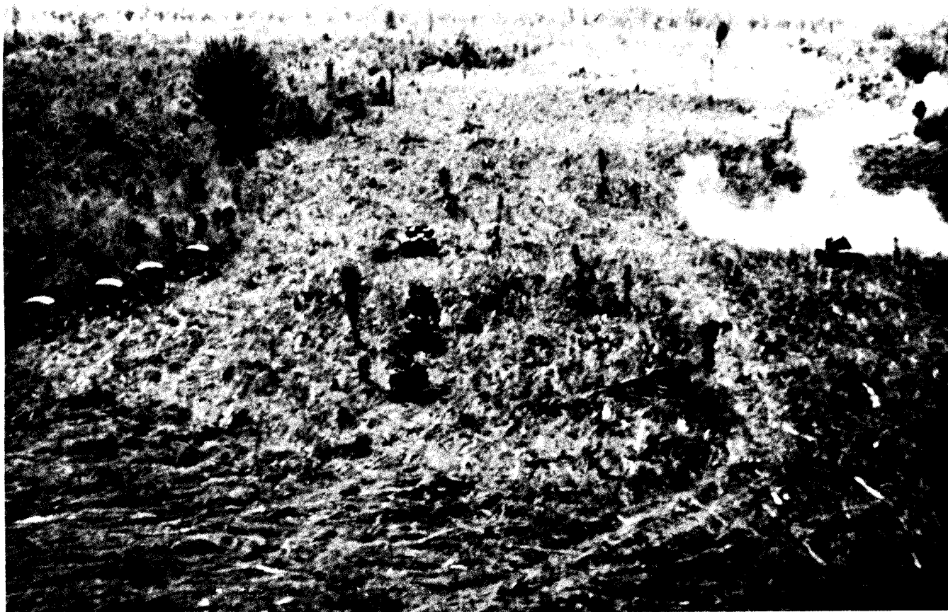
Figure 2-4. Area clearing in a tactical operation. Note. Isolated large trees are left standing.
