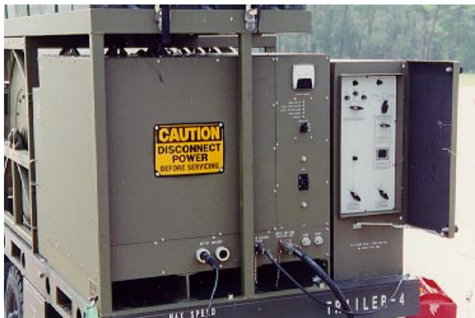
Figure 9.20. EALS Regulator and Control Panel.
