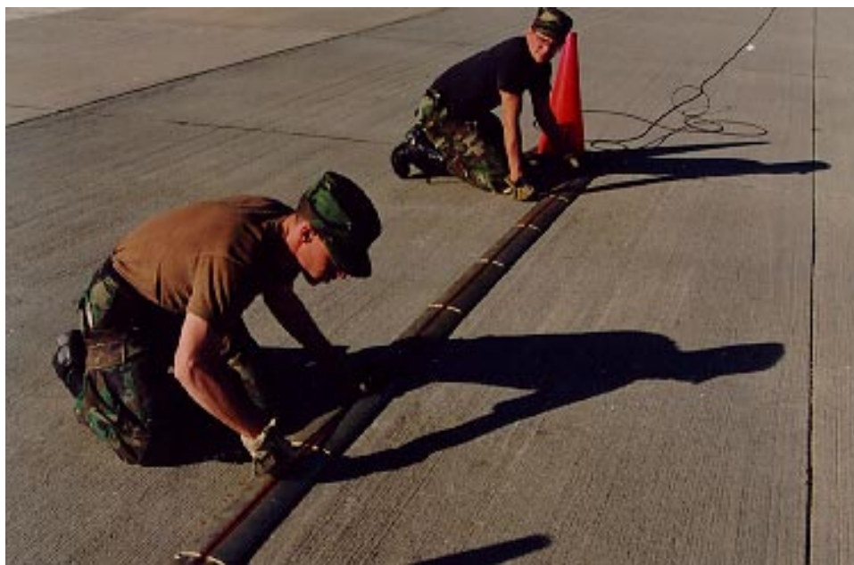
Figure 9.19. EALS Cable Protectors.
