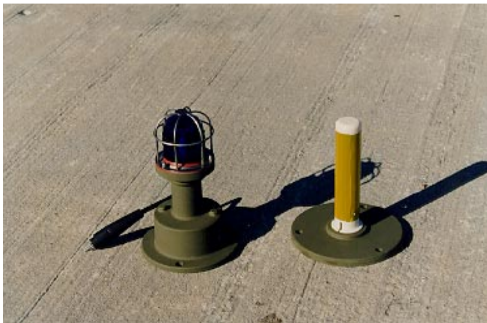
Figure 9.14. EALS Taxiway Lights.
