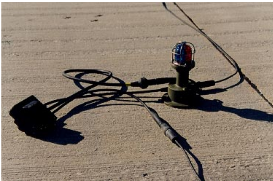
Figure 9.13. EALS Threshold and End Lights.
