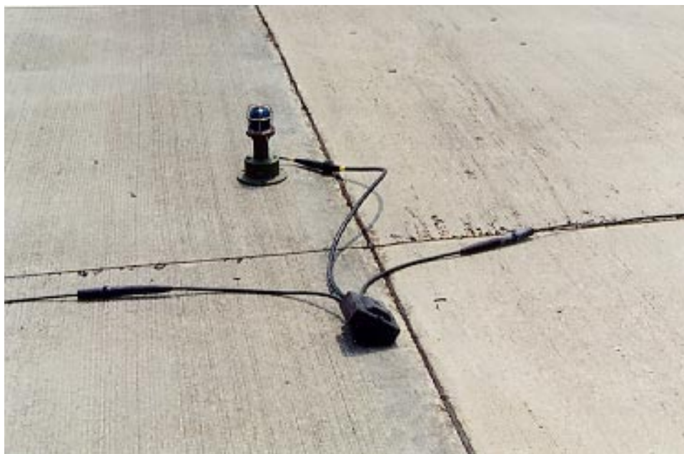
Figure 9.15. EALS Isolation Transformers.
