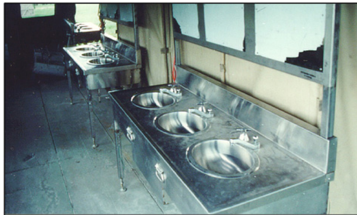
Figure 21. Shower/Shave Unit Sinks.
