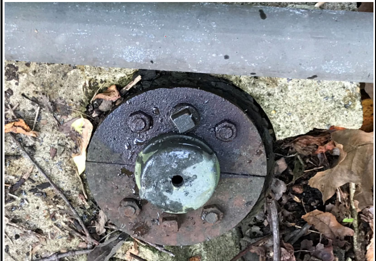
Photo 2. S19496 Former Barracks well and emergency supply well
