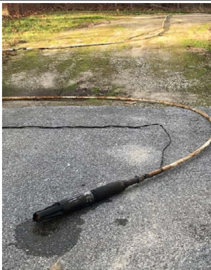
Photo 1: Pump and feeder tube removed from S 19495.
