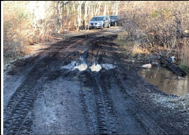
Photo 1. Ruts in the access path to Old Montauk Highway caused by vehicle traffic. USACE and AECOM will discuss restoration of the roadway with the State Park Superintendent.
