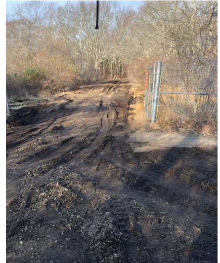
Photo 6. Access roadway to new monitoring wells after application of gravel and smoothing of ruts with Bobcat (TWS/ADT).
