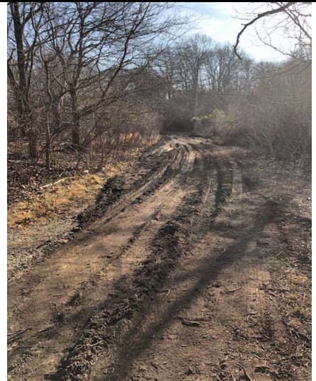
Photo 8. Access roadway to new monitoring wells after application of gravel and smoothing of ruts with Bobcat (TWS/ADT).
