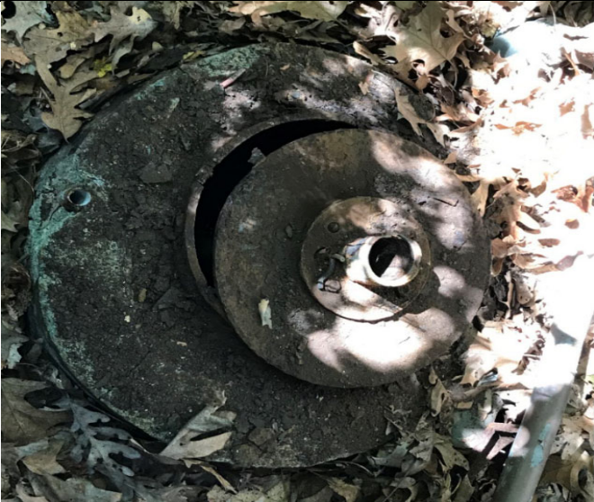
Photo 3. Supply well S21084 in pump house western perimeter of Camp Hero
