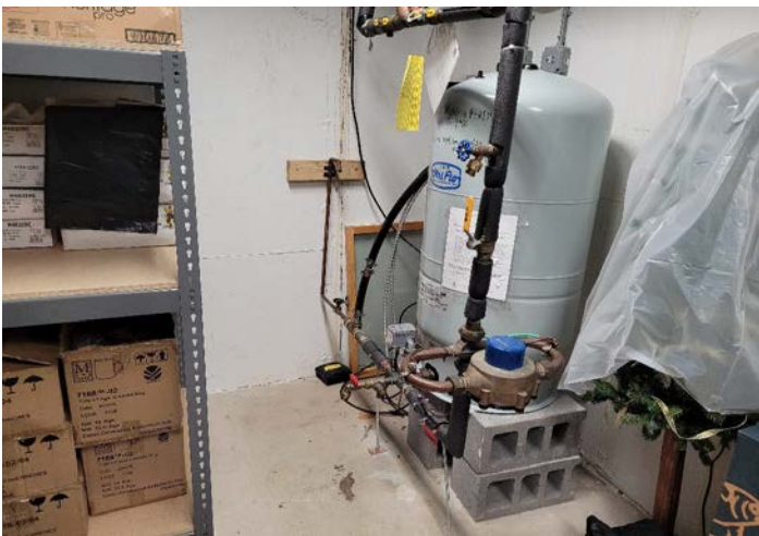
Photo 1. Giftshop water supply system; influent sample port identified.
