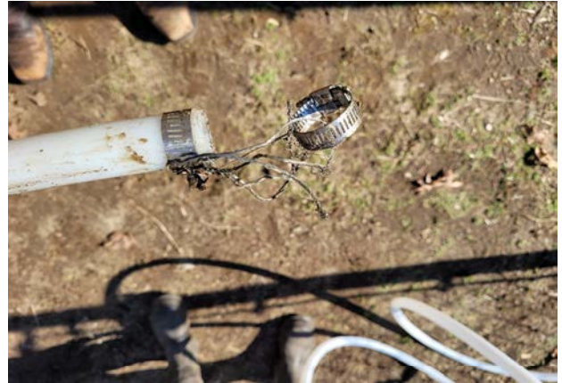
Photo 4. Failed check valve security during well redevelopment at S76304 (Madison Hills Well 1).
