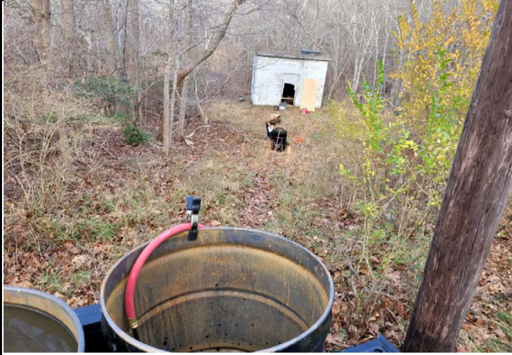
Photo 1. Well redevelopment at S 17231S (Former USAF Supply Well; inside pump house).
