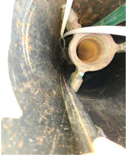
Photo 5. Inside S 121811 (Madison Hill Well 3A)
